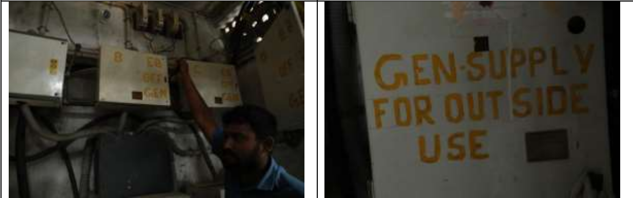
Power control Board
