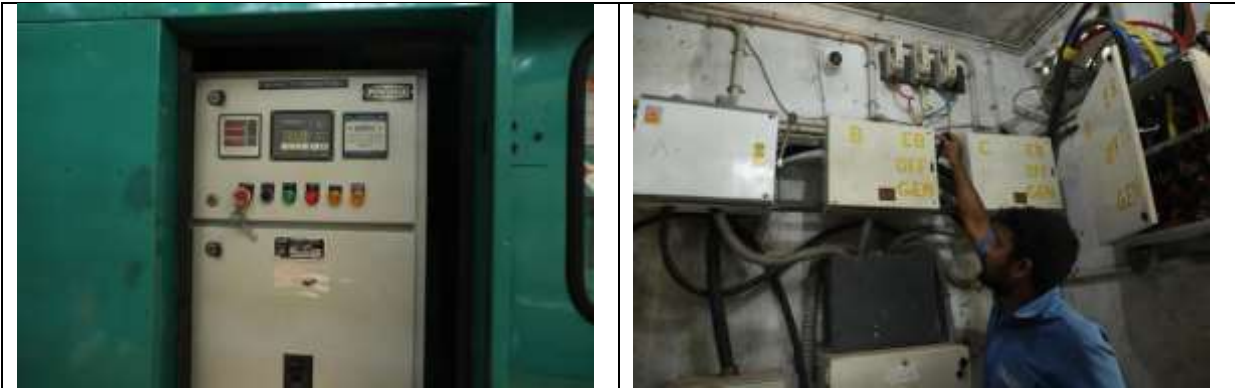
DG Set Control Unit
