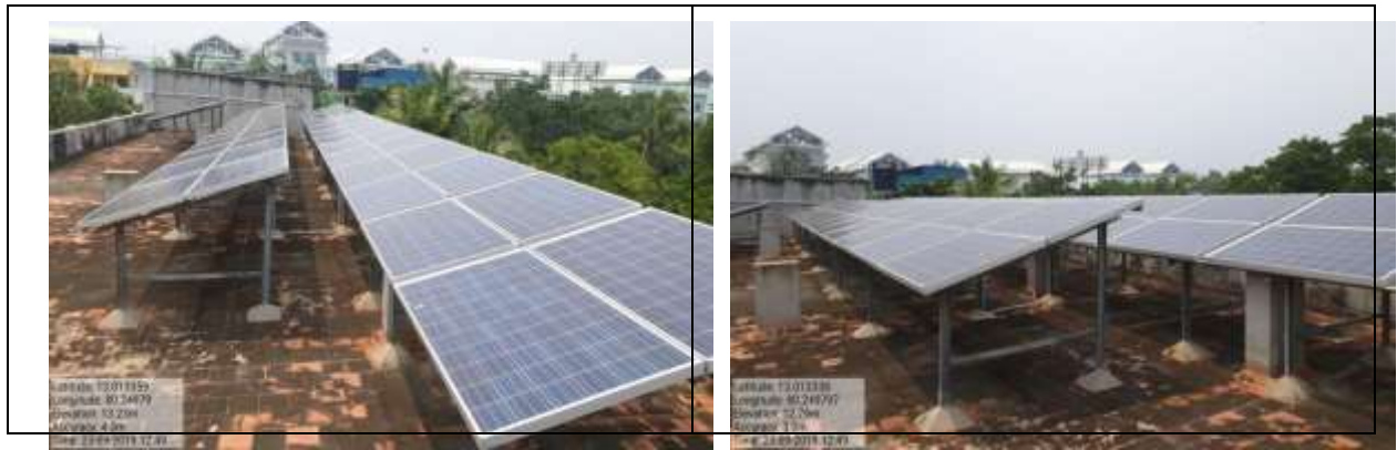
Solar Panels – B Block
