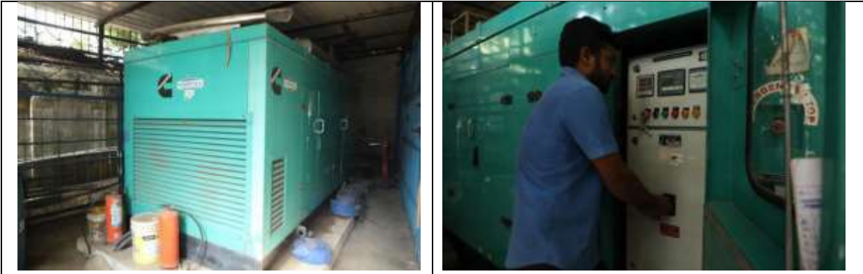
Diesel Generator Set
